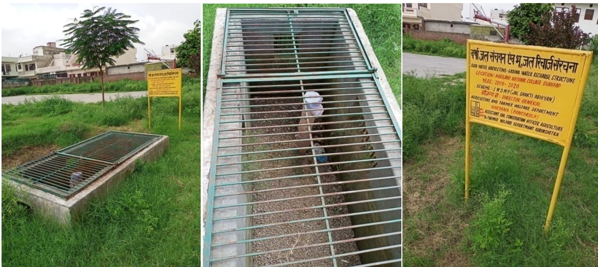
Water Harvesting Plant
