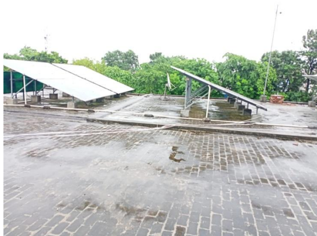
20 KV SOLAR POWER PLANT
